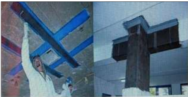
Fig 1: A) Application of Externally Bonded FRP Composites. B). Retrofitting Of Column-Beam Joint
