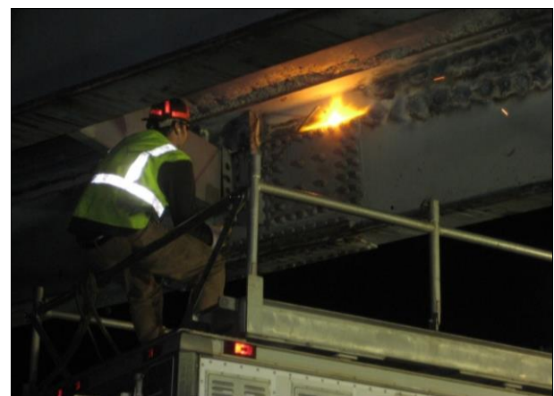
Fig 5: Line heat on the web of the girder
