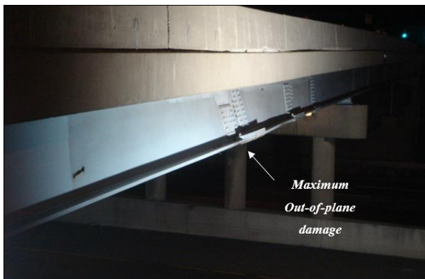
Fig 2: Damage on Allisonville Road Bridge
