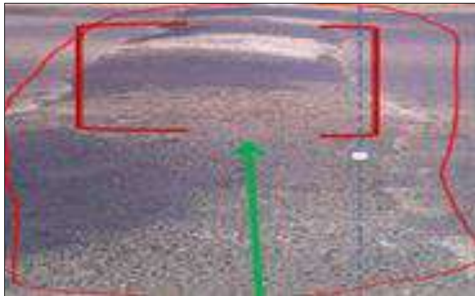
Fig 6: Unsuitable speed breaker on Combolcha – Dessie road
