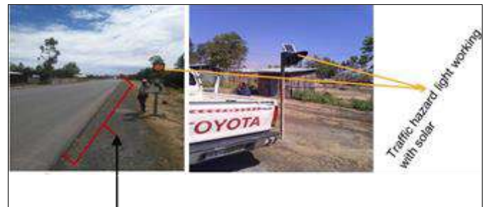
Fig 5: Intervention made at Sebeta – Tulu Bolo road (traffic hazard light).
