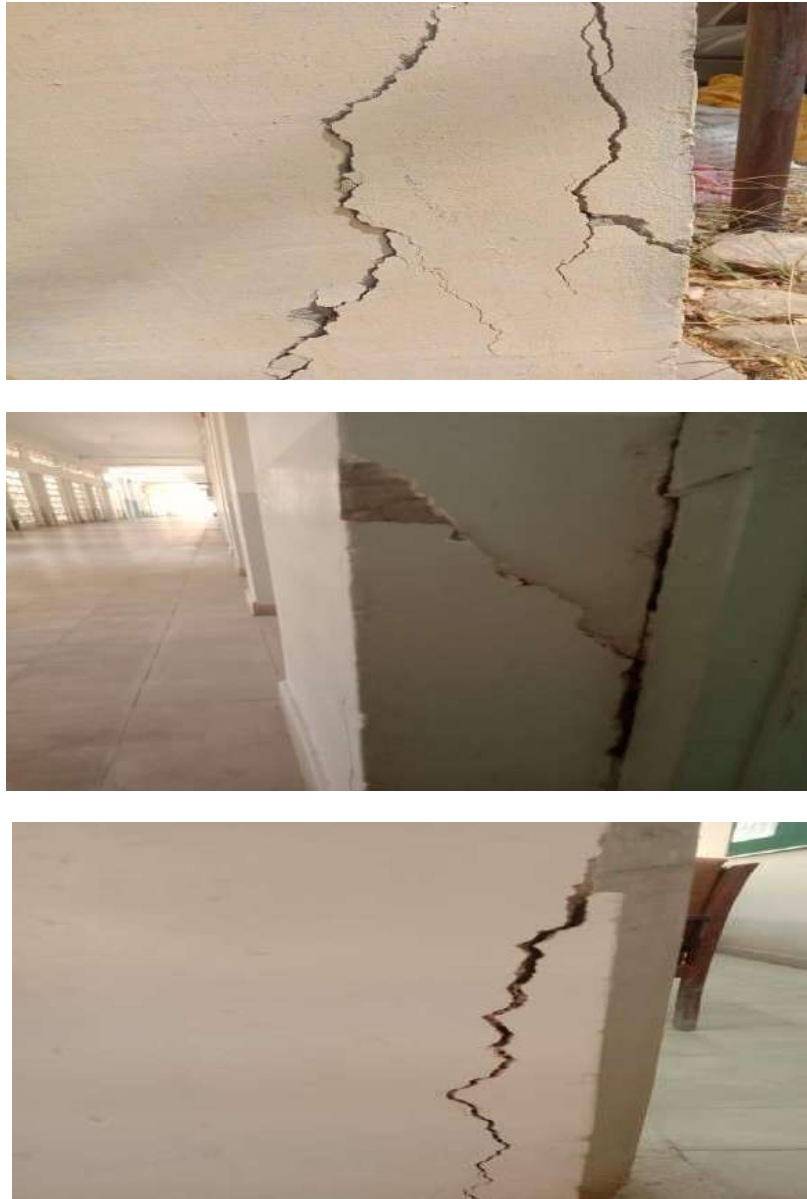
Fig 2: Cracks showing size and orientations in the building
