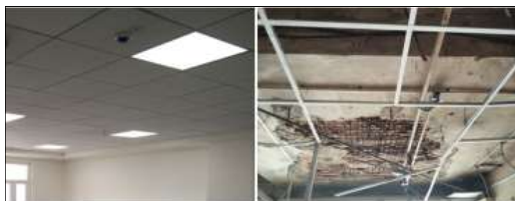
Fig 3: Sunken slab with false ceiling and without false ceiling
