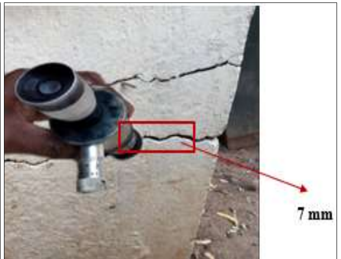
Fig 10: Location L 7, Crack width 70 mm
