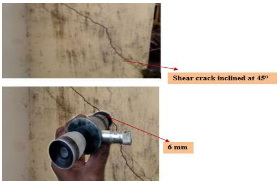
Fig 8: Location L 5, longitudinal Shear crack length >1000 mm, crack width= 6 mm.
