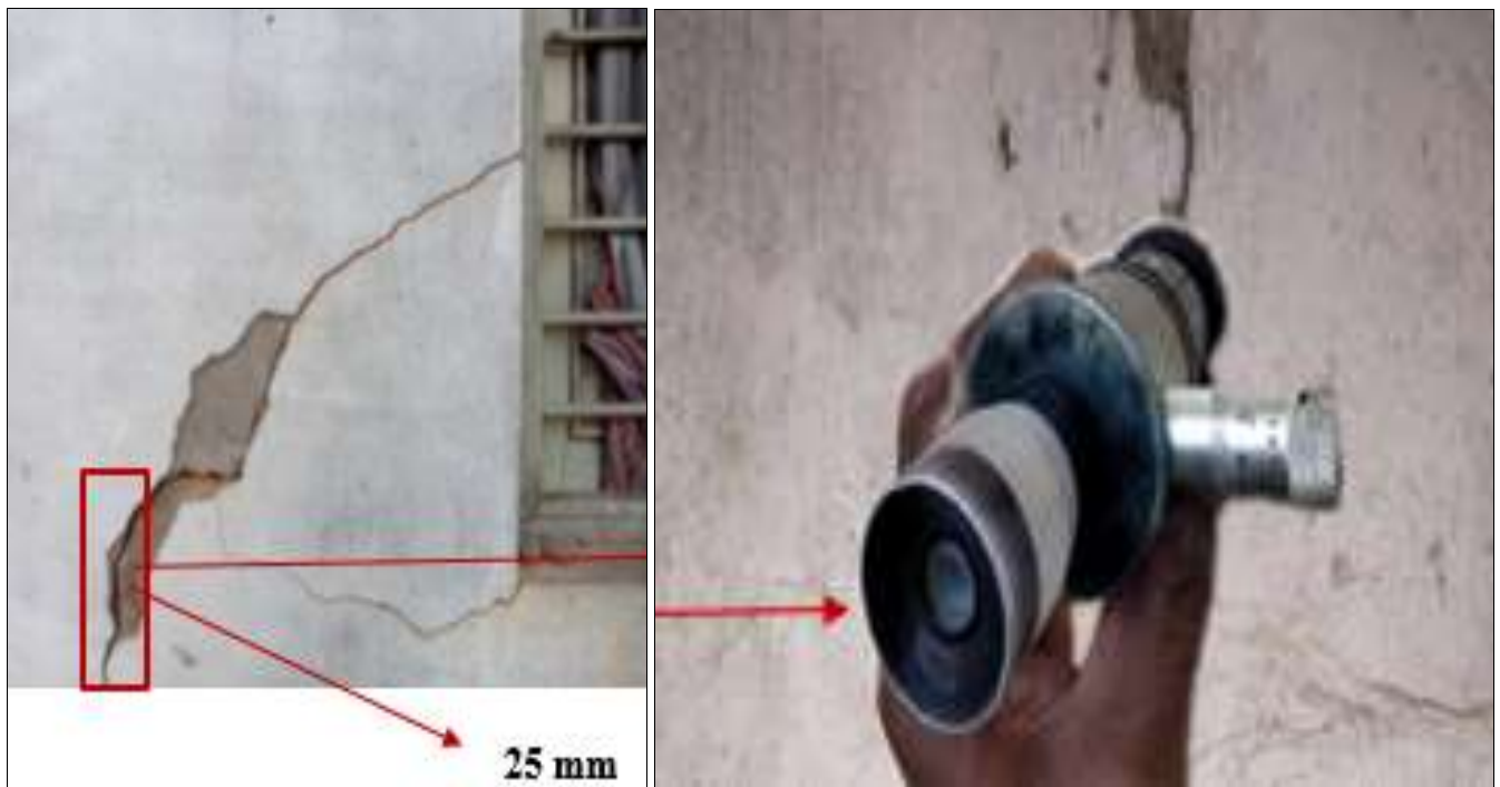
Fig 11: Location L 8, Crack width 25 mm and 1000 mm length
