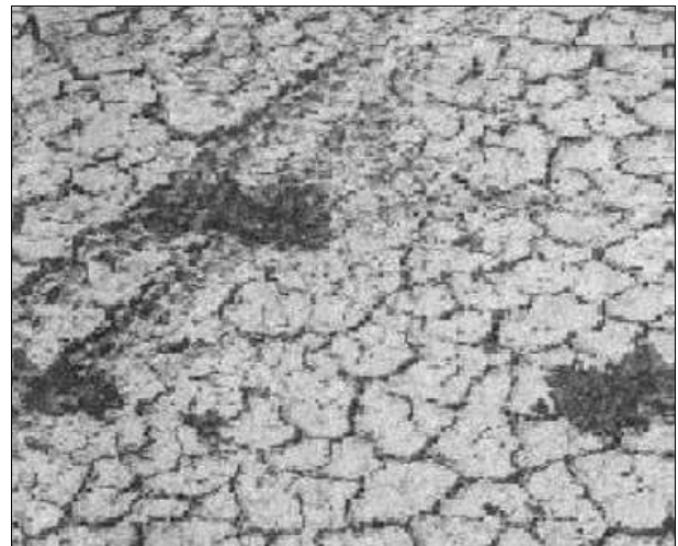
Fig 1: Expansive soil with cracks
