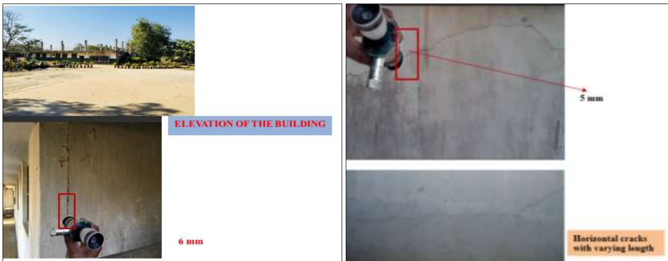
Fig 7: Location L 3, crack separates the wall and column Fig 8 location L 4, longitudinal cracks in the main wall
